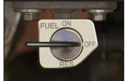
FUEL SUPPLY VALVE IN OFF POSITION
